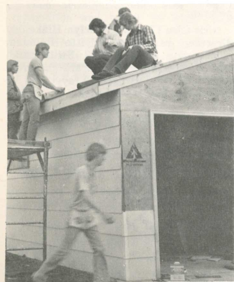
This two stall garage is being built by members of the building construction class under the direction of instructor Glen Everson for one of the local lumber companies and is designed to give practical experience for members of the class.
